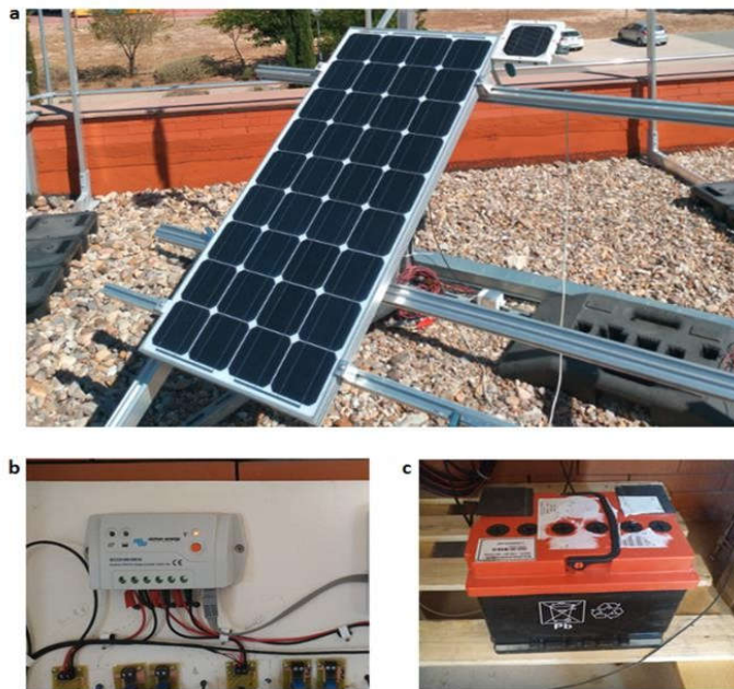
Figure 6 SAPV System Installed at IMDEA Water Institute Facilities: PV Mono- Crystalline Module (a), Charge Controller (b) and Lead-Acid Battery (c).
