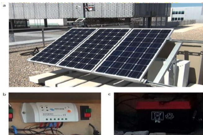
Figure 7 SAPV System Installed at University of Linares Facilities: PV Mono- Crystalline Module (a), Charge Controller (b) and Lead-Acid Battery (c)
